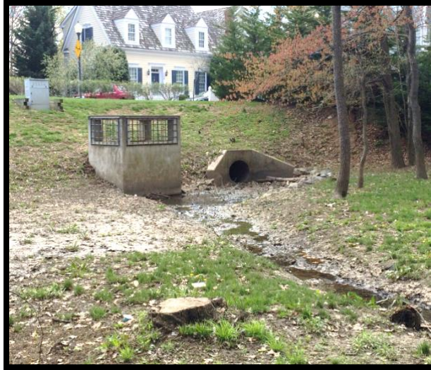
Inlet storm drain pipe and outlet riser structure at Kentlands stormwater dry pond facility.
