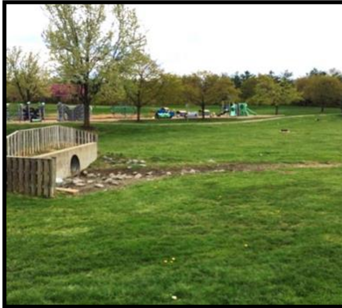
Existing outfall to Green Park dry pond shows evidence of sediment and trash debris
