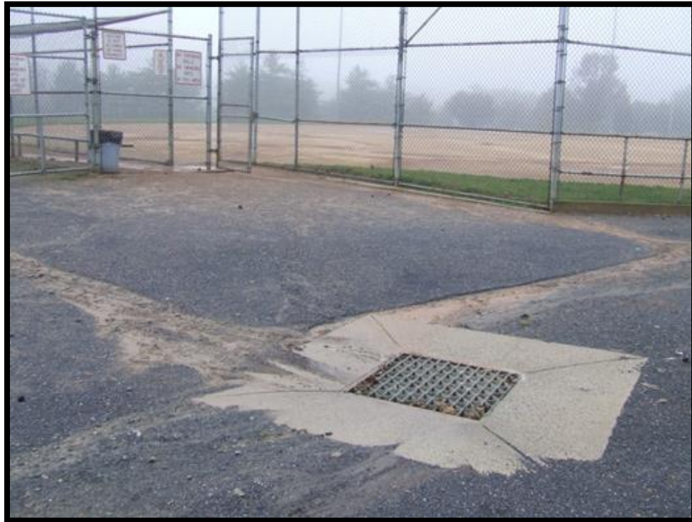
Gravel and sediment entering a storm drain at Kelley Park
